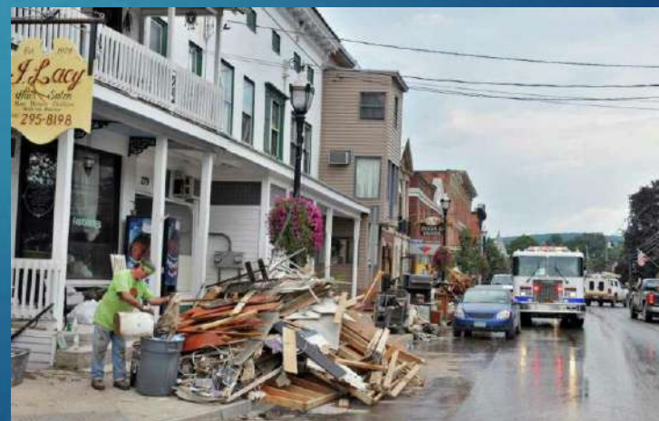
Main Street, 2011 Flood Clean-up
